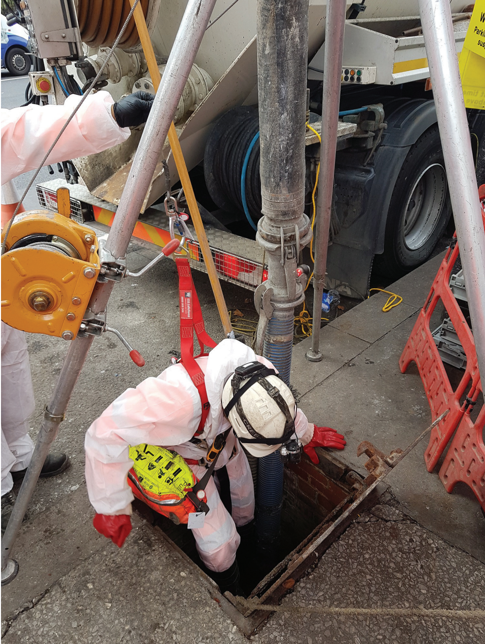
The fatberg had to be broken down into pieces small enough to fit a manhole. This hard manual work was described as sewer workers fighting a dangerous and disgusting monster. Photo: Thames Water.
